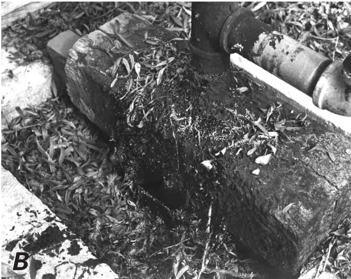
Figure 10.—The Peck well in Los Gatos, Calif. (figs. 1, 5). A , Well and pump unit within a fenced enclosure in a parking lot. B , Black oily substance on pipe and wooden block at wellhead; part of casing is just barely visible in center beneath wooden block. Sample of oil was obtained from about 3.7-m depth by lowering a glass jar through narrow space between well casing and wooden block.
