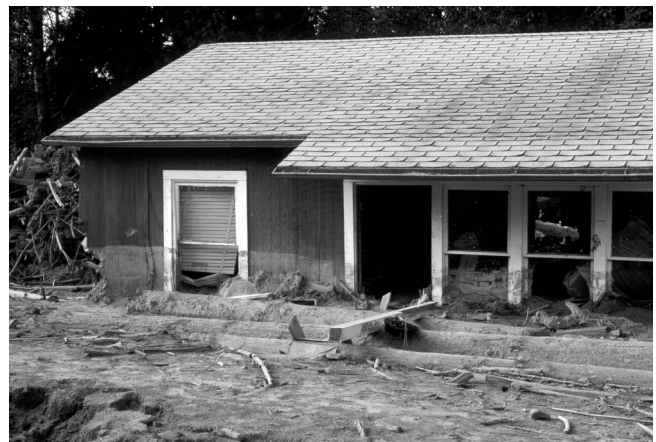
Figure 6. This house in a distal hazard zone of Mount St. Helens was partly buried by lahars from the 1980 eruption. Note the high mud line on the house and large amounts of woody debris carried by the lahars. Photo by Lyn Topinka, USGS.
